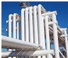
Industrial Gases Pipeline
