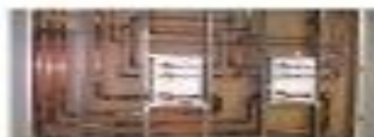
Medical Gas Pipelines
